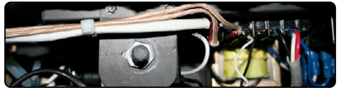
Figure 4.g Control box controls
